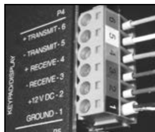
Photo 3.17—Terminal Strip P4 Wiring Connection on the SSC1500 Control Module
