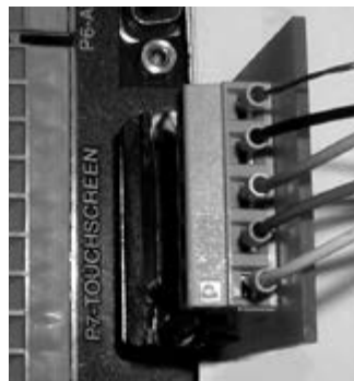
Photo 3.20—P7 Touchscreen Port Wiring Connection on the Main CPU Card
