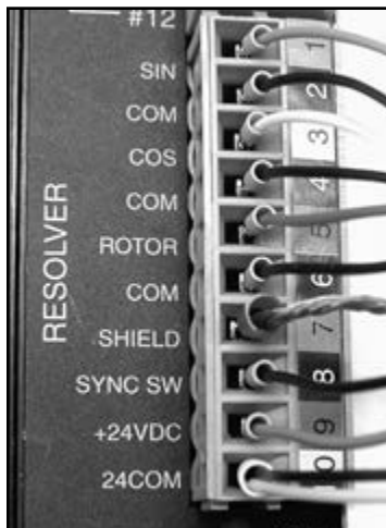
Photo 3.26—Terminal Strip P8 Wiring Connection on the SSC3000 Main CPU Card
